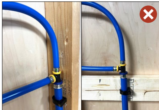
Figures 9.12a & 9.12b INCORRECT Fastening Locations that will Cause Excessive Stress on Joints at Fittings
