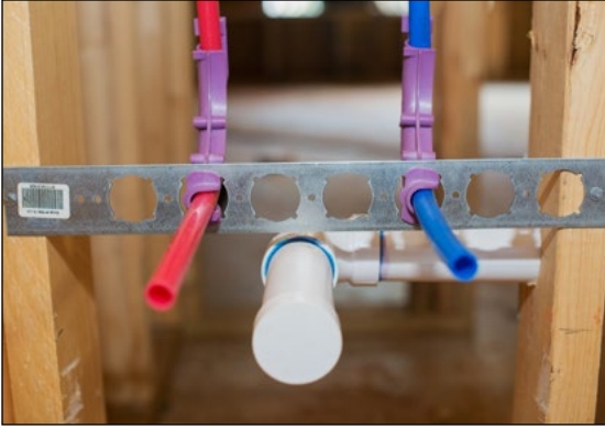
Figure 9.41 PEX Tubing Run Through the Wall to a Plumbing Fixture
