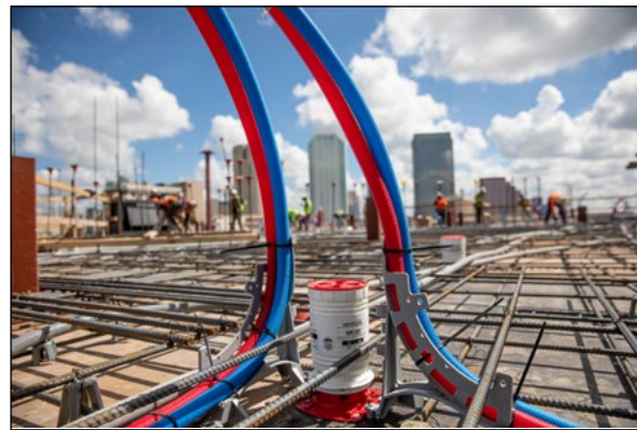
Figure 9.31 PEX Tubing Held Vertically when Emerging from a Slab Using Special Guides
