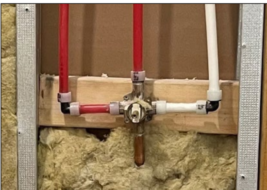
Figure 9.48 PEX Tubing Connected to a Shower Valve in 3 Locations
