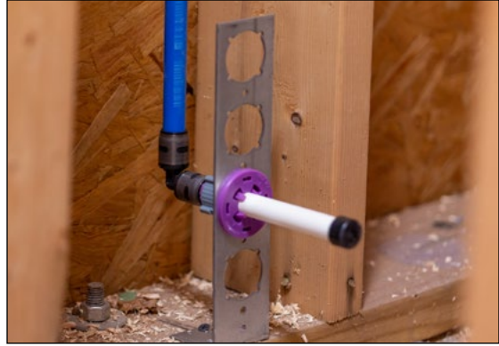
Figure 9.42 PEX Tubing Run Through the Wall to a Plumbing Fixture
